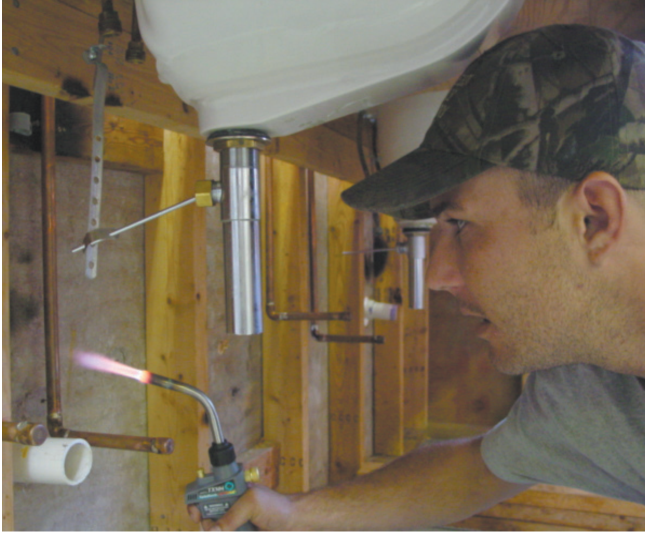
Plumbers often go between the walls of homes or commercial buildings to install or repair plumbing systems, fixtures, and appliances.
