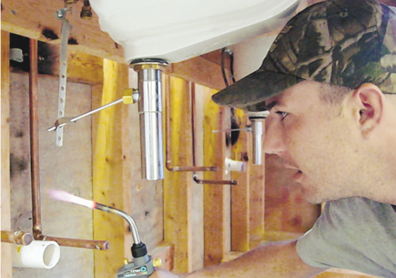
Plumbers often go between the walls of homes or commercial buildings to install or repair plumbing systems, fixtures, and appliances.
